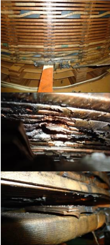
Figure-7 Failure of Winding
