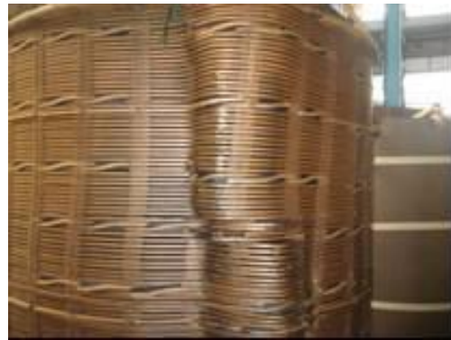
Figure-6 Damaged winding of Transformer
